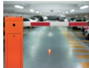
ATV12 controlling an access barrier
